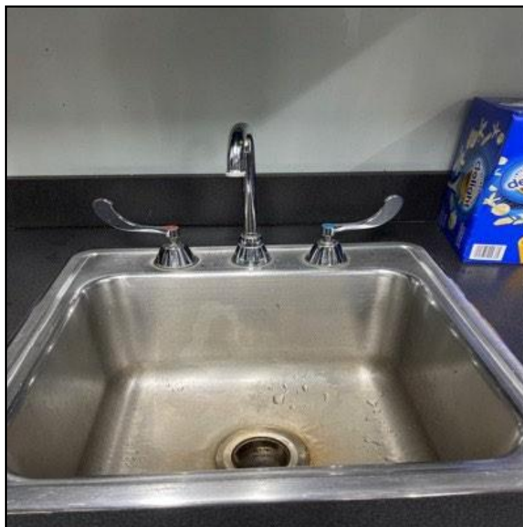
View of potential DWO and sample 02-02-225-DW-P-29
