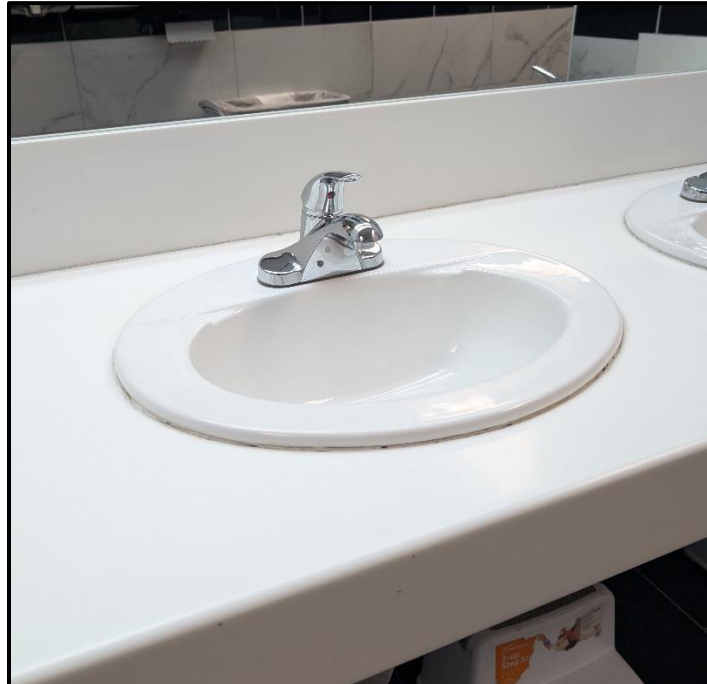
View of potential DWO and sample 02-01-00H-BF-P-6 (Initial sample taken following notice of repairs. Outlet was offline during September 13, 2023 sampling.)
